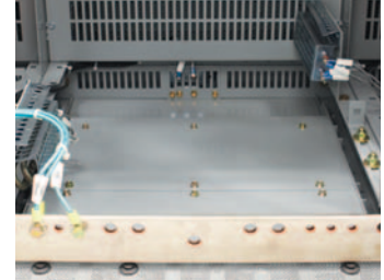
Cable Compartment Floor Plates
